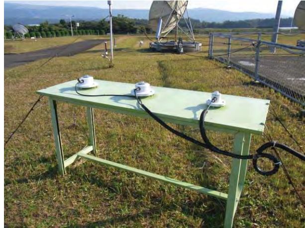
Figure 1 Photograph of solar radiation monitoring system installed at Tokai University Space Information Center.
